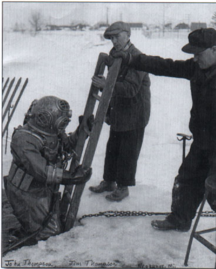
John, on ladder, and Jim Thompson (center) at work on a municipal water line in Negaunee, Michigan.
