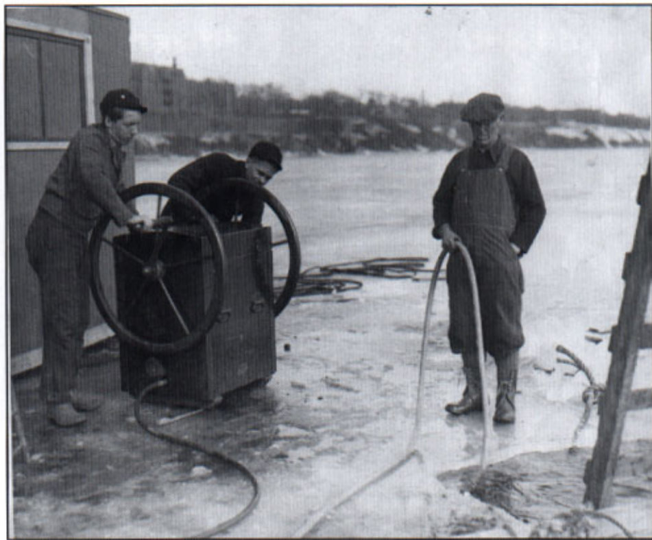
Capt. Horace H. Thompson tends the air line for his son John Thompson, below, while Howard Geisert and Frank Smith man the pumps. They are laying a water line in Lake Superior for the Fitger company off Duluth's Sixth Avenue East in 1935.
